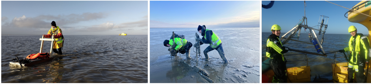
Figure 2. Photographs illustrating the installation of the measurement stations. Left: transport of instruments and equipment to intertidal measurement locations, after vessel grounding. Middle: in situ assembly of a scaffold frame equipped with instruments on a fringing mudflat. Right: deployment of an instrumented lander from a vessel.
