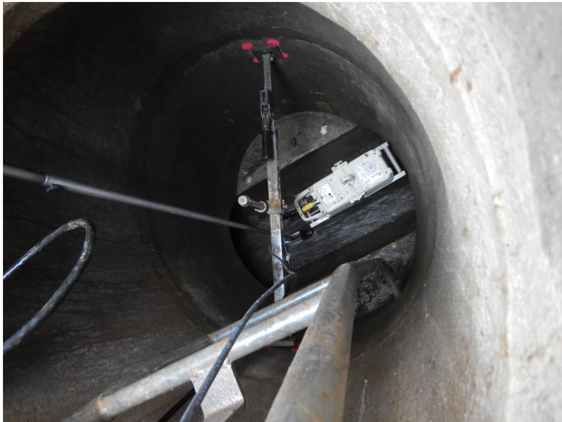
Figure S 25: Flo-Dar installed in manhole during comparison with portable flow meter
