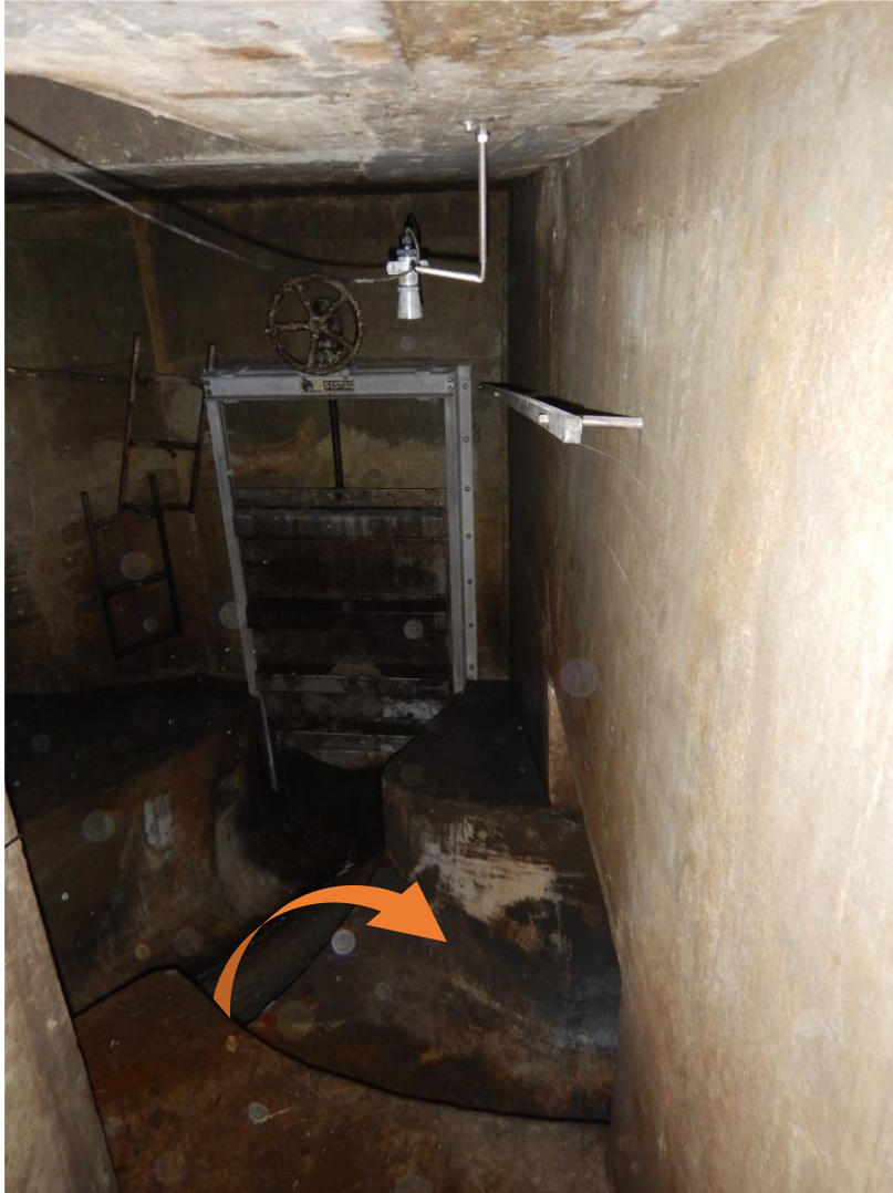
Figure S 16: Flow splitter VS22 with a manually operated gate at the outlet. The arrow indicates the possibility of in-sewer overflows diverting the sewage to RU 40a (photo taken from HBT 2016).
