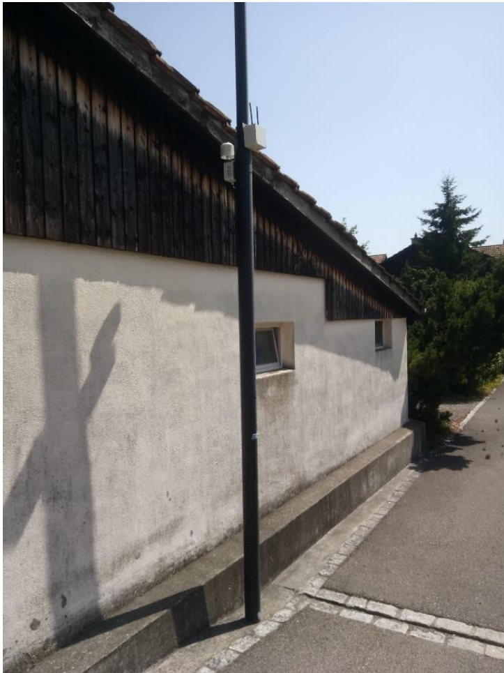
Figure S 30: LoRa-Mesh repeater node (upper box) self-sufficient with the Solar Panel
