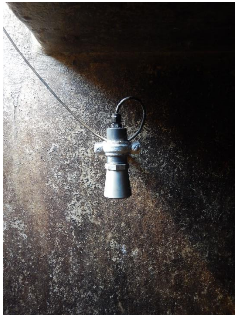
Figure S 22: Example installation of the rugged water level sensor Maxbotix sensor in the sewer. The cable makes it possible to place the sensor in a different spot at the monitoring site than the logger. This is important to optimize both sensor performance and data transmission.
