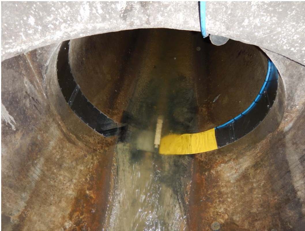
Figure S 27: Nivus POA correlation wedge sensor(barely seen on the ground) inside the sewer
