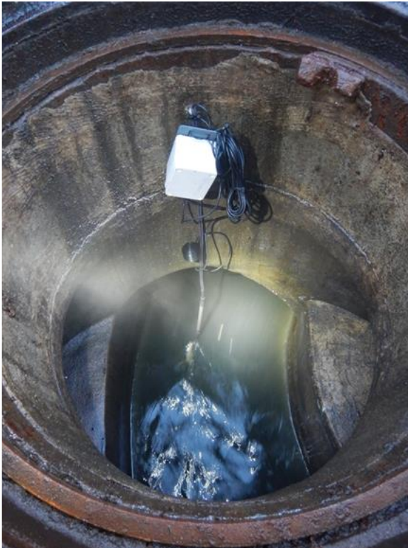
Figure S 24: Example installation of a dual temperature sensor, which simultaneously record temperatures of the wastewater and the sewer atmosphere.
