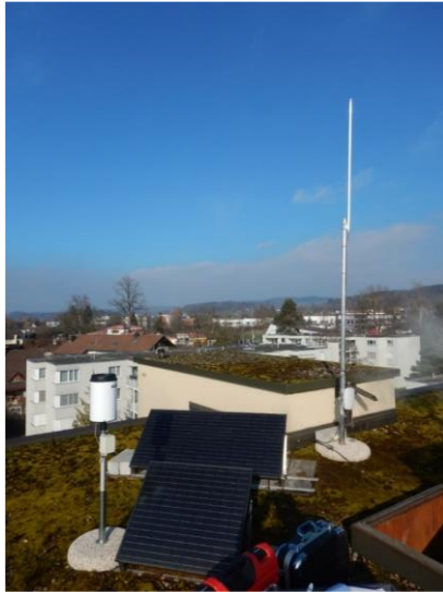
Figure S 34: Gateway at the rooftop of a high rise building, including solar panels powering the entire system.
