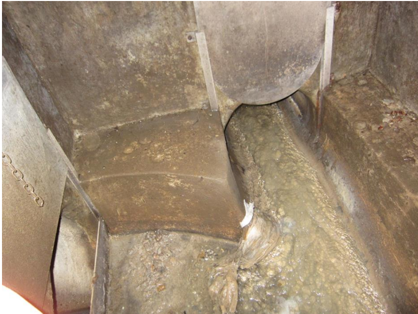
Figure S 15: Flow splitter VS600 with slide gates (photo taken from the GEP – HBT, 2016).
