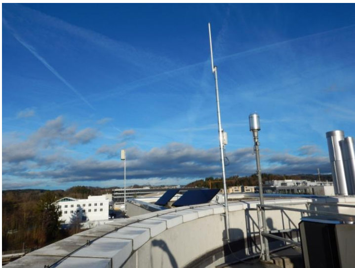
Figure S 35: Gateway at the rooftop of the Fehrlortorf WWTP control building.
