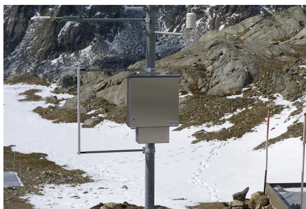
Figure 10. The SND snow drift sensor installation at the Bella Vista AWSS. The sensor elements are placed in the cylindrical tube that is vertically held in place by two mounting arms building a rectangular shape (left of the logger box). In the background (lower left in the photo), the snow scale in the slight depression is visible (sheltered site, sink for snow deposition). The snow pillow besides the main AWSS mast (lower right in the picture) measures SWE at the exposed location.
