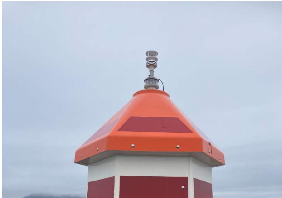
Figure 2. Weather station installed on top of the Gåsøyane lighthouse.
