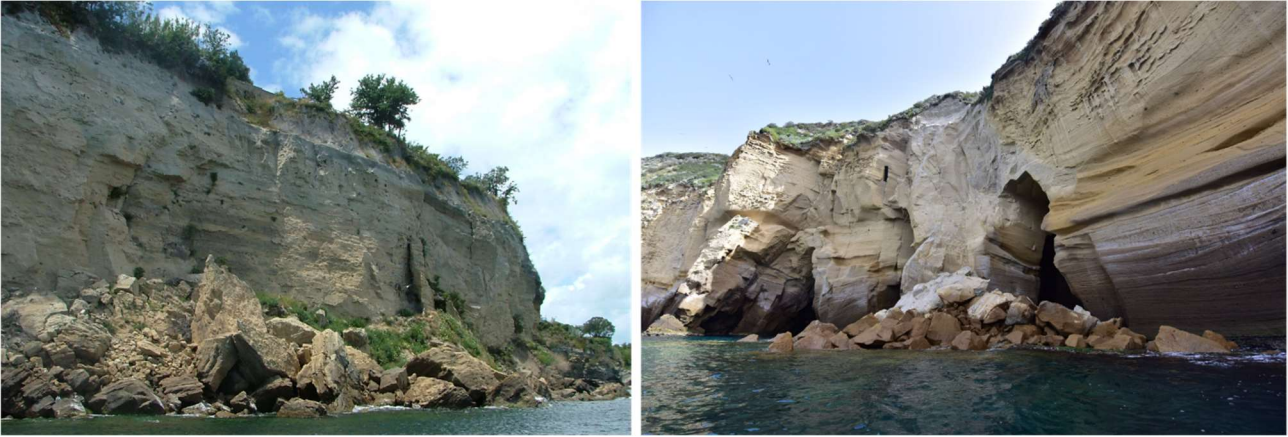
Figure 45: Examples of rock fall affecting the Campi Flegrei coastal cliffs: Punta Miseno (2015) on the left, and Trentaremi - Capo Posillipo (2017) on the right (both sites are indicated in Fig. 1). (Image credits: Alessandro Fedele, INGV).
