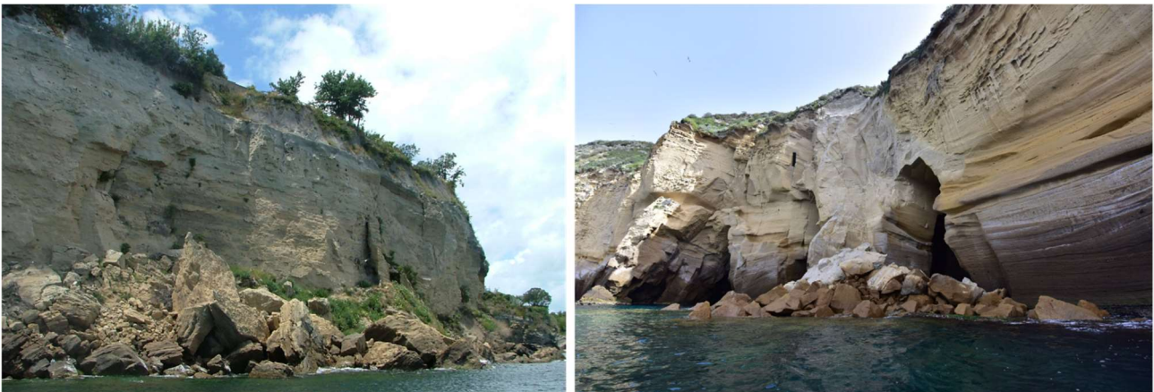
Figure 4: Examples of rock fall affecting the Campi Flegrei coastal cliffs: Punta Miseno (2015) on the left, and Trentaremi - Capo Posillipo (2017) on the right (both sites are indicated in Fig. 1) . (Image credits: Alessandro Fedele, INGV).
