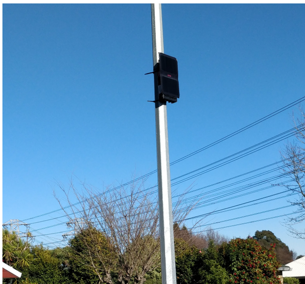
Figure 4. An example of a typical ODIN installation on a light-pole.
