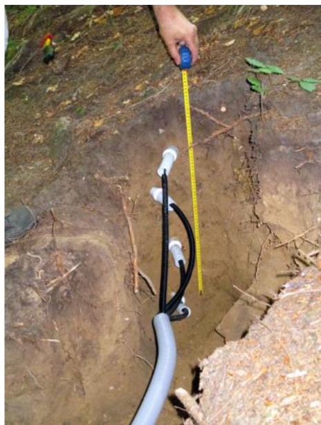
Figure 4: HydraProbe sensors installed at site Q2S0
