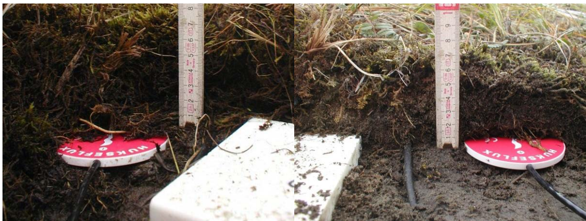
Figure B12. Hukseflux HFP01 ground heat-flux sensors ( left: center, right: rim ), installed on 24 August 2002.
