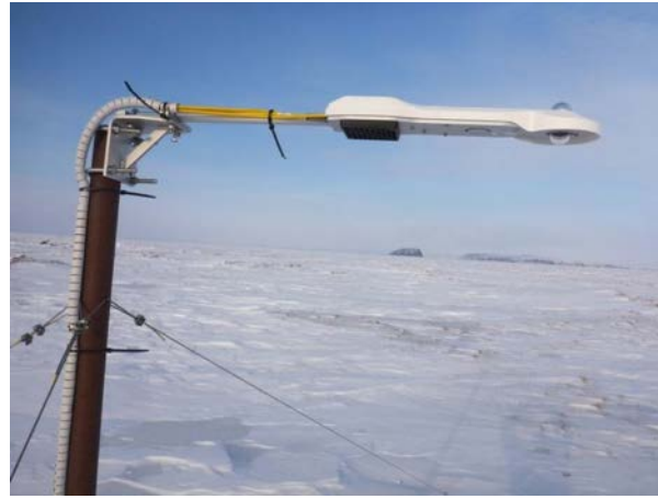
Figure B3. Kipp & Zonen CNR4 radiation sensor (including CNF4 ventilation unit) for measuring incoming and outgoing shortwave and longwave radiation, respectively, installed on 22 August 2014.
