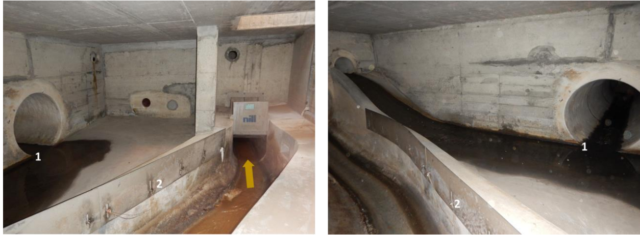
Figure S18. Overflow chamber RU 40a with slide gates (photos taken from HBT, 2016; modified). The left and right pictures show a downstream and upstream view. The numbers 1 and 2 label same points of reference and the arrow indicates downstream flow direction.
