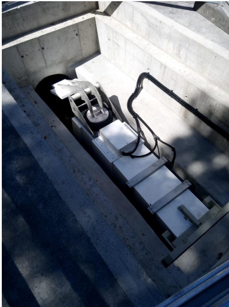
Figure S29. Pneumatic flow limiter, partially-filled, at the main collector just upstream of the WWTP inlet.
