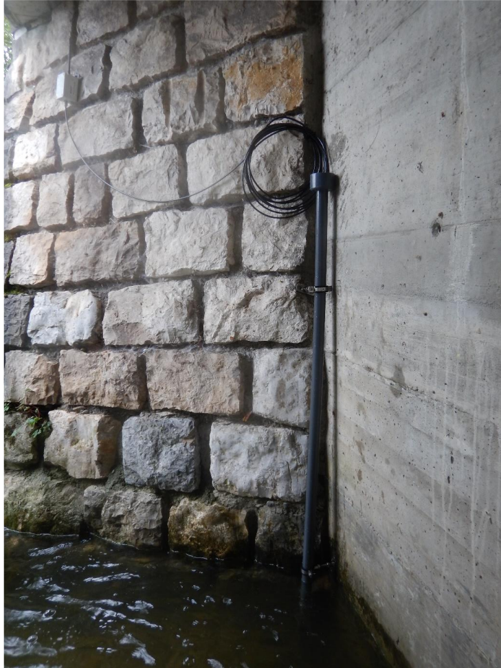
Figure S27. Pressure probe inside a protective hull connected with the LoRaWAN-logger
