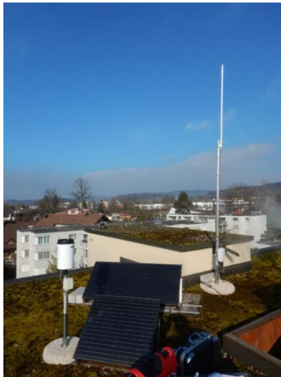
Figure S32. Gateway at the rooftop of a high rise building, including solar panels powering the entire system.
