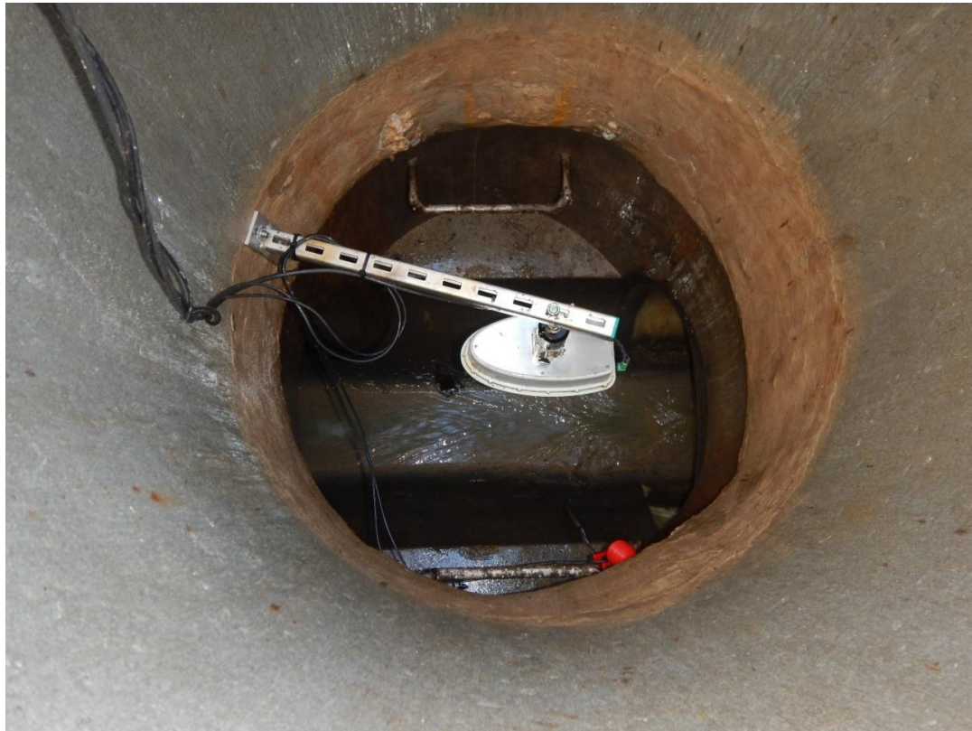
Figure S24. Sommer SQ-3 flow meter in a “low-flow” measurement site.
