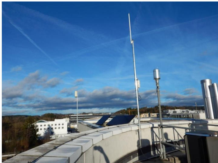
Figure S33. Gateway at the rooftop of the Fehraltorf WWTP control building.
