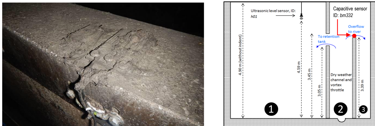
Figure S47. Left: Capacitive sensor for overflow discharge detection at the weir crest basin RUB 59 after three years of operation. Photo: S. Bloem, Eawag. Right: Cross-section through overflow structure (not drawn to scale). including inflow chamber (2), retention tank (1), overflow to receiving water (3) and US level sensor (h01) and the capacitive sensors (bm332 and dl311).
