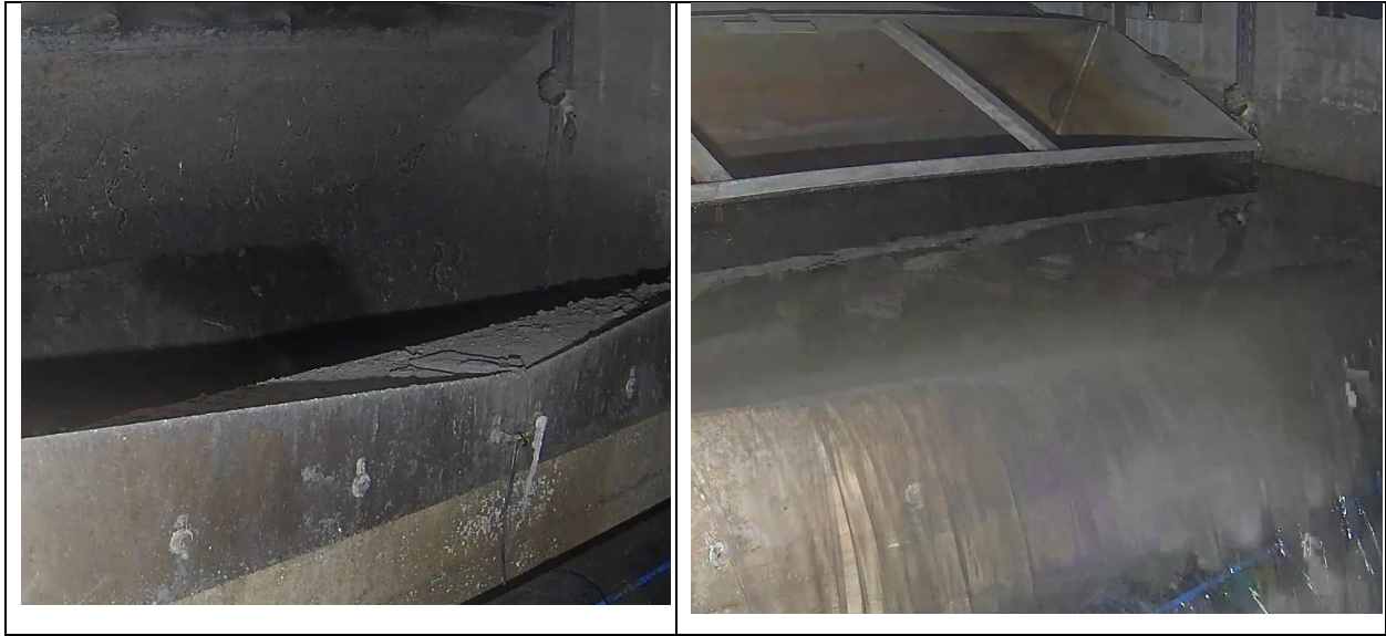
Figure S22. Left: the Decagon sensor, i.e. Meter 5TM mounted on a weir crest in dry environment; right: submerged sensor in case of an overflow event.
