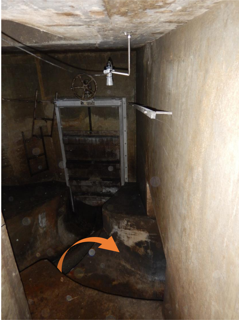
Figure S17. Flow splitter VS22 with a manually operated gate at the outlet. The arrow indicates the possibility of in-sewer overflows diverting the sewage to RU 40a (photo taken from HBT 2016).
