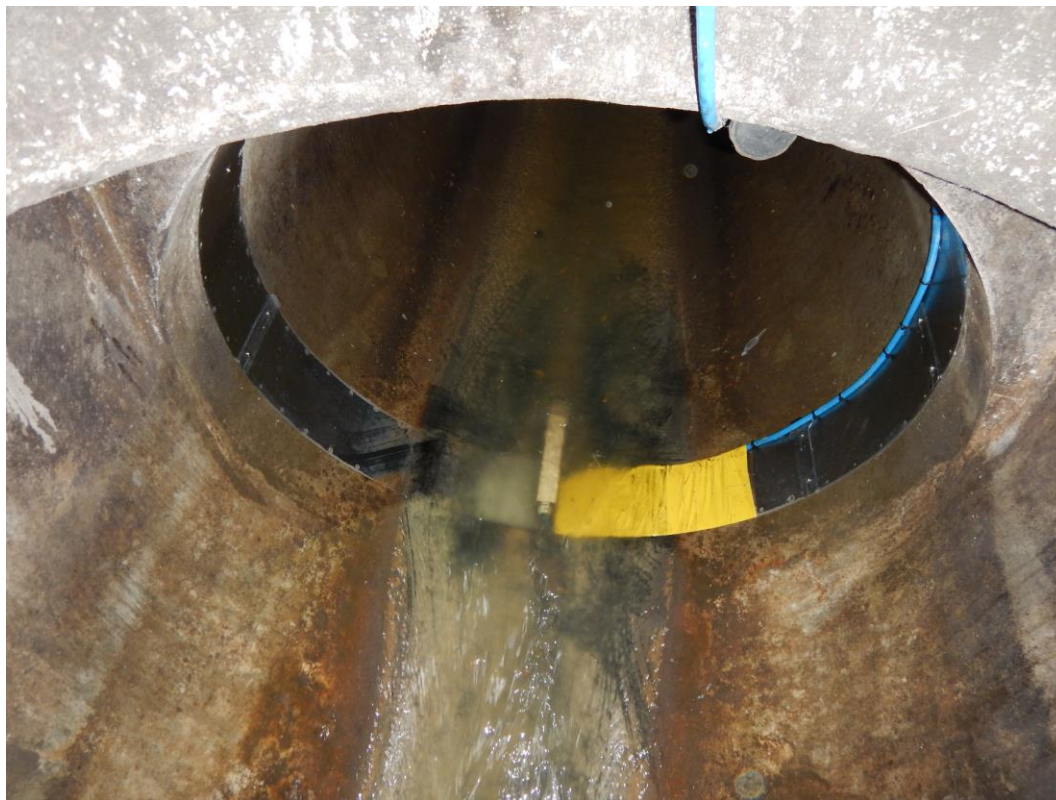
Figure S25. Nivus POA correlation wedge sensor(barely seen on the ground) inside the sewer
