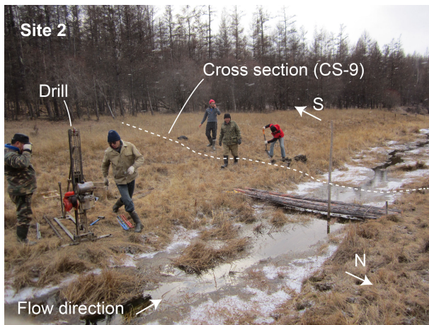
Figure D2. Installation of HOBO thermistor chains, and piezometer tubes at Site 2 (CS-9) with a petrol powered standing drill.
