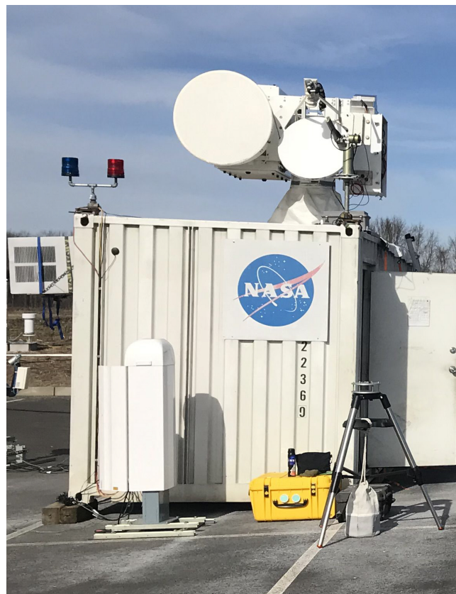
Figure 7. Deployment of the ACHIEVE trailer with the W-Band Radar on the roof during 2022–2023 at the D3R site.
