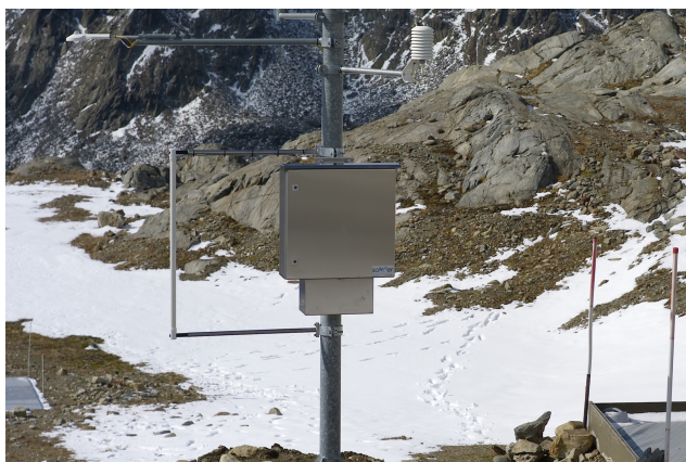
Figure 10. The SND snow drift sensor installation at the Bella Vista AWSS. The sensor elements are placed in the cylindrical tube that is vertically held in place by two mounting arms, building a rectangular shape (left of the logger box). In the background (lower left in the photo), the snow scale in the slight depression is visible (sheltered site, sink for snow deposition). The snow pillow beside the main AWSS mast (lower right in the picture) measures SWE at the exposed location.
